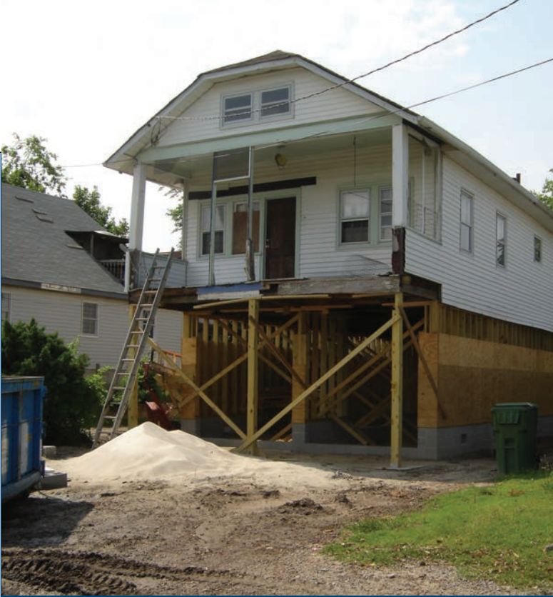
A Norfolk house being raised due to chronic flooding on 51st Street.
